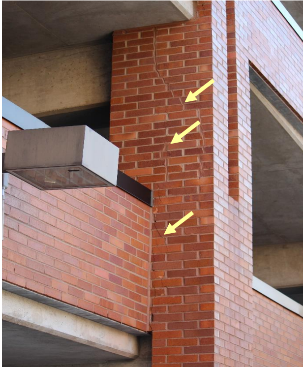
Figure 7. Distress at Column 19A prior to brick removal.
