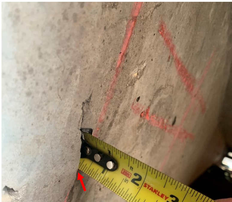
Figure 12. Approximately 1/4" displacement across crack in original concrete at Column 11A.
