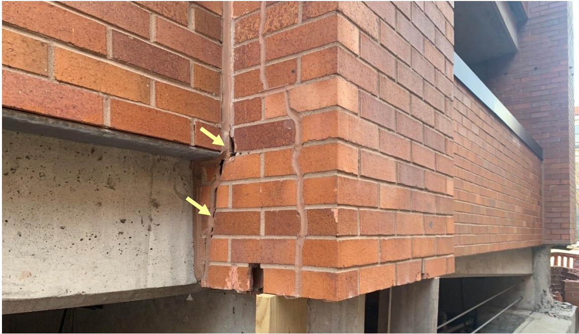
Figure 17. Cracks propagating through previous sealant repairs in the brick veneer at Column 11A.
