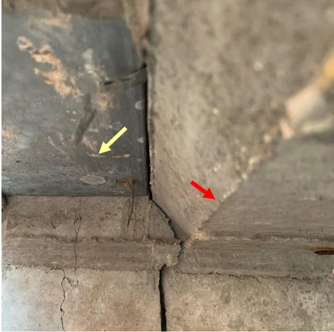
Figure 15. Crack in original concrete at south face of Column 11A extends along slab edge bearing at column. Slab indicated with red arrow and shelf angle indicated with yellow arrow.
