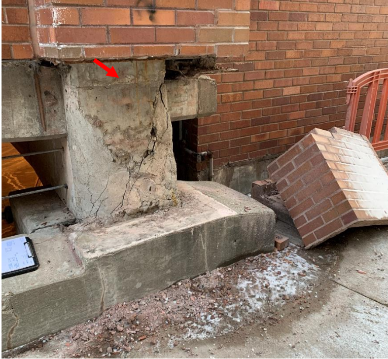
Figure 3. Brick veneer removed from the base of Column 10A. A steel shelf angle supporting the brick veneer indicated with red arrow.
