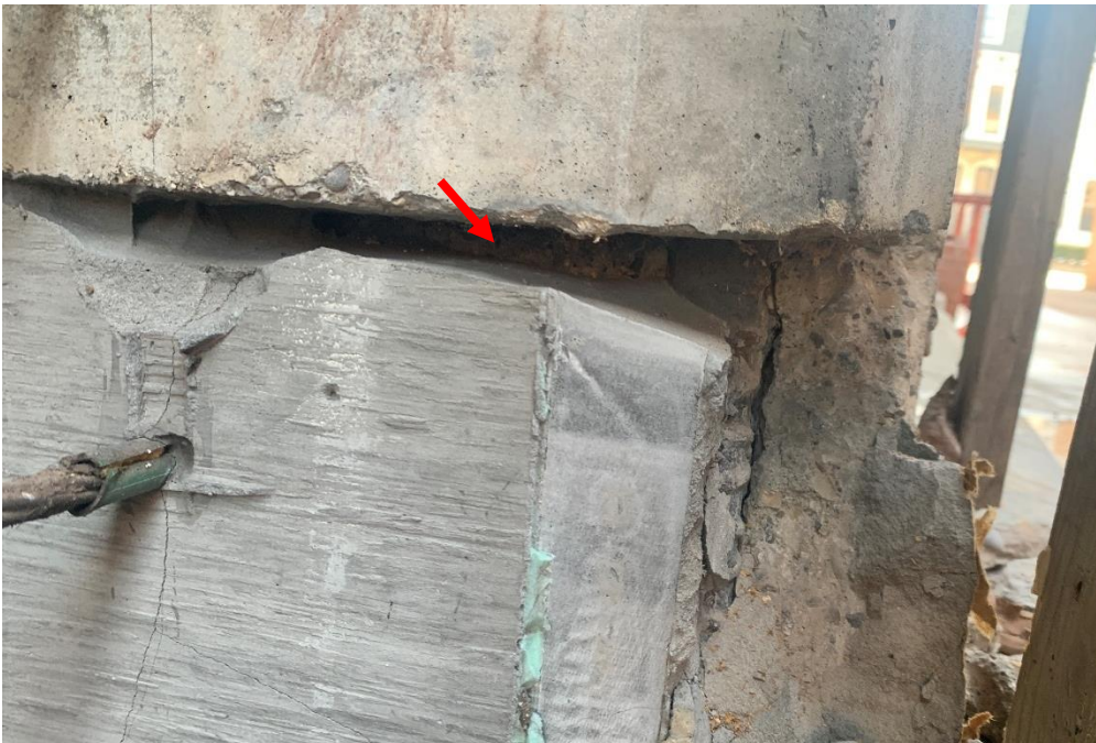
Figure 16. Wide cold joint at north face of Column 11A between original concrete and concrete repair. Joint is approximately four inches deep.
