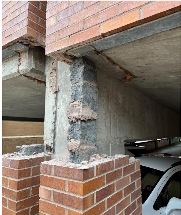
Figure 4. Column 19A inspection opening at Level 2 PT beam end (brick veneer at concrete block infill removed).
