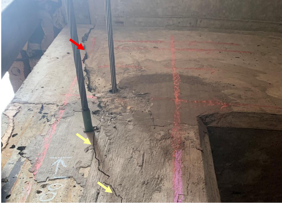
Figure 11. Cracks throughout concrete at Column 11A. Crack propagates through original concrete above as indicated with red arrow. Note the displacement across the crack in the original concrete where the concrete material has spalled.
