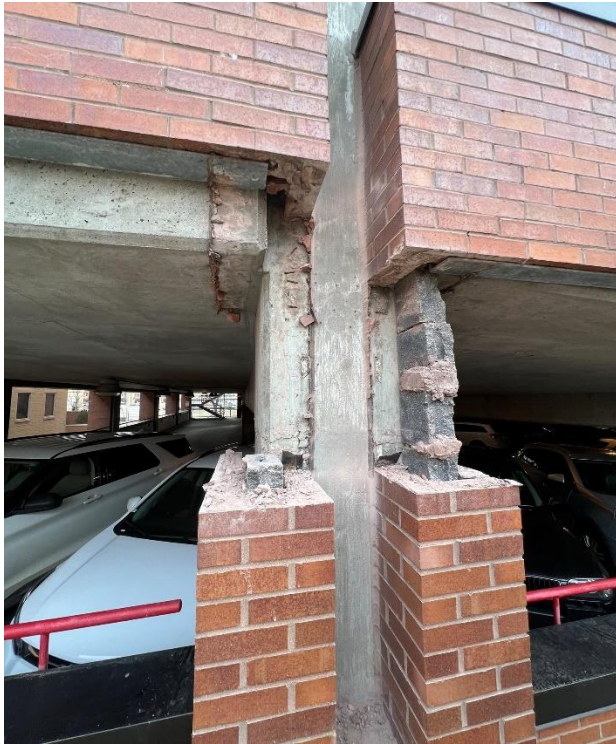
Figure 3. Column 19A inspection opening at Level 2 PT beam end (brick veneer at concrete block infill removed).
