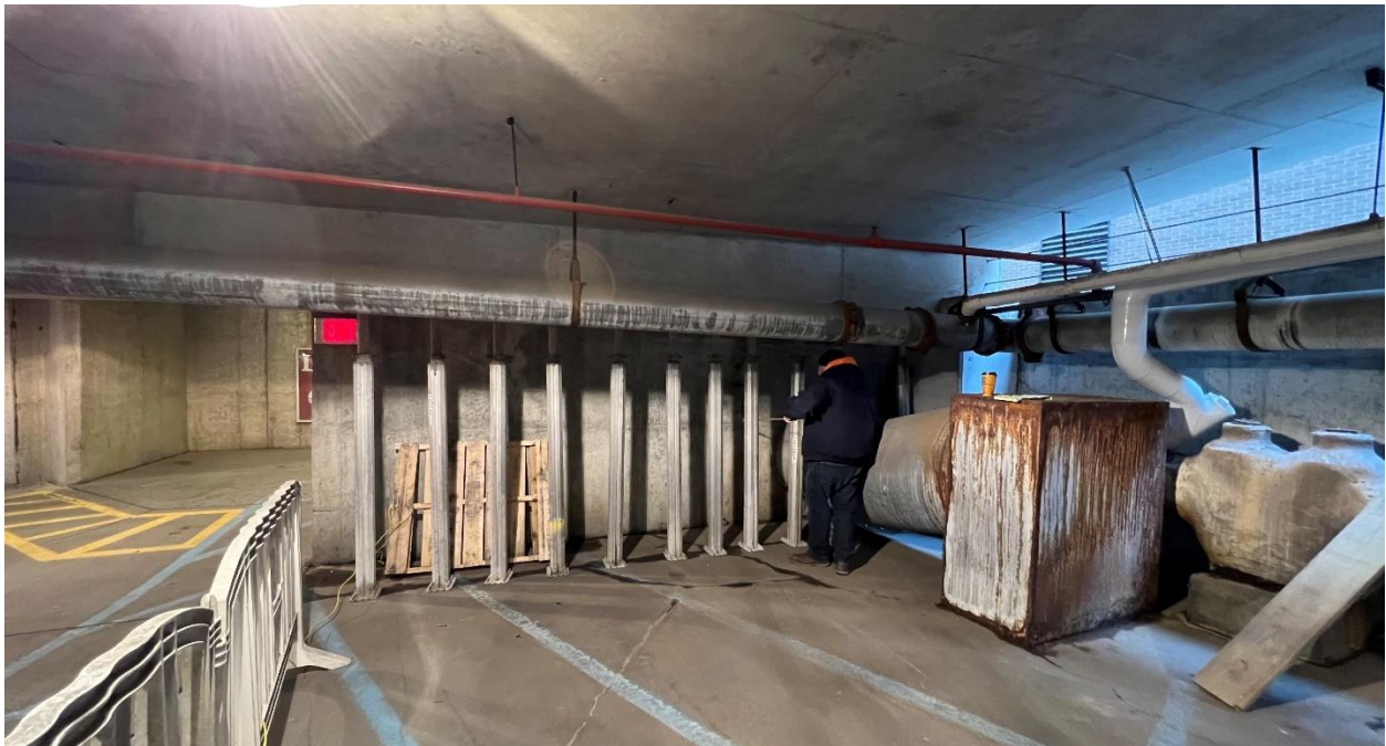
Figure 2. Shoring posts installed at the west end of the Level 1 beam supported by Column 10A.
