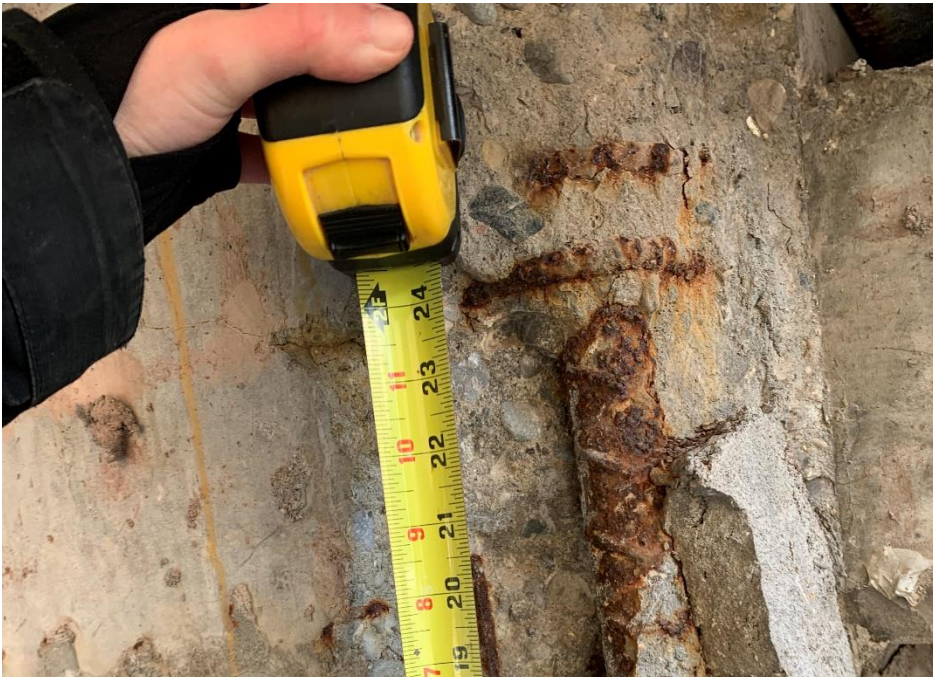
Figure 6. 24 inches from curb to first exposed stirrup at Column 10A.
