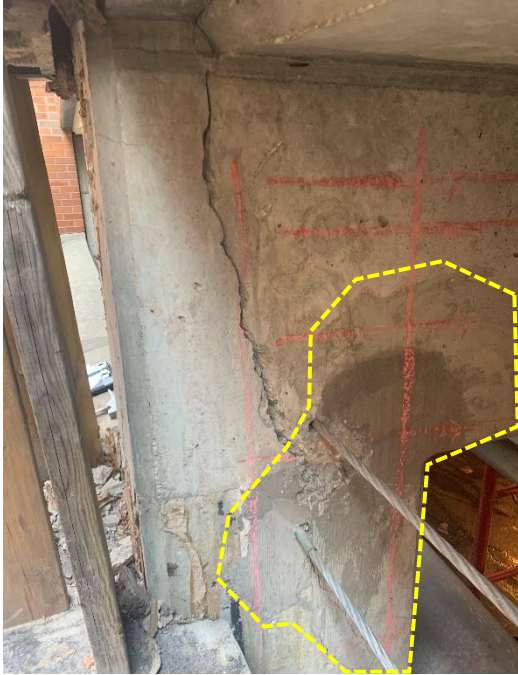
Figure 9. Previous concrete repair at beam to column interface at south face of column.
