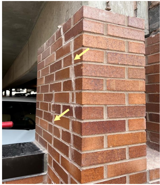
Figure 6. Brick distress below the existing inspection opening at Column 19A.
