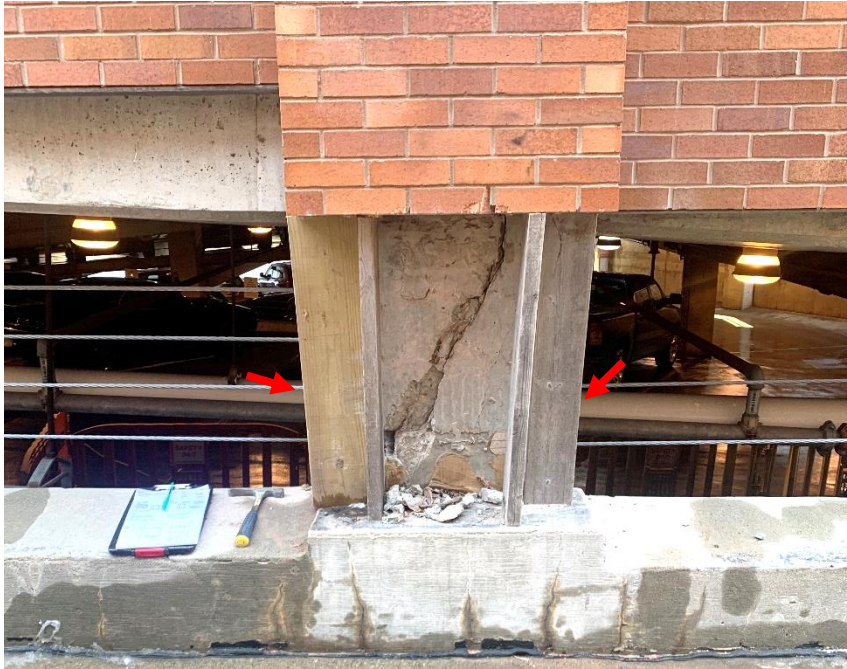
Figure 8. Brick veneer removed at Column 11A (west face) and supported by wood framing indicated with red arrows.
