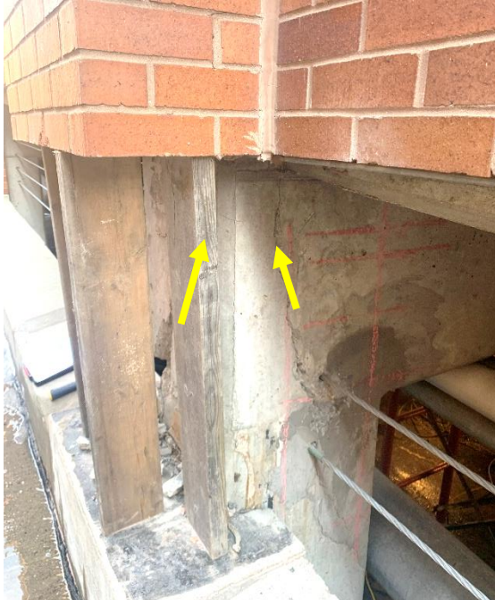
Figure 14. Cracks in west and south faces of Column 11A extend toward a converging point.
