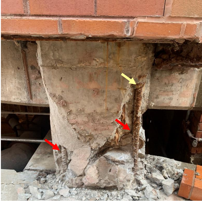
Figure 5. #11 longitudinal bars at corner of Column 10A are indicated with red arrows. Stirrup indicated with yellow arrow.
