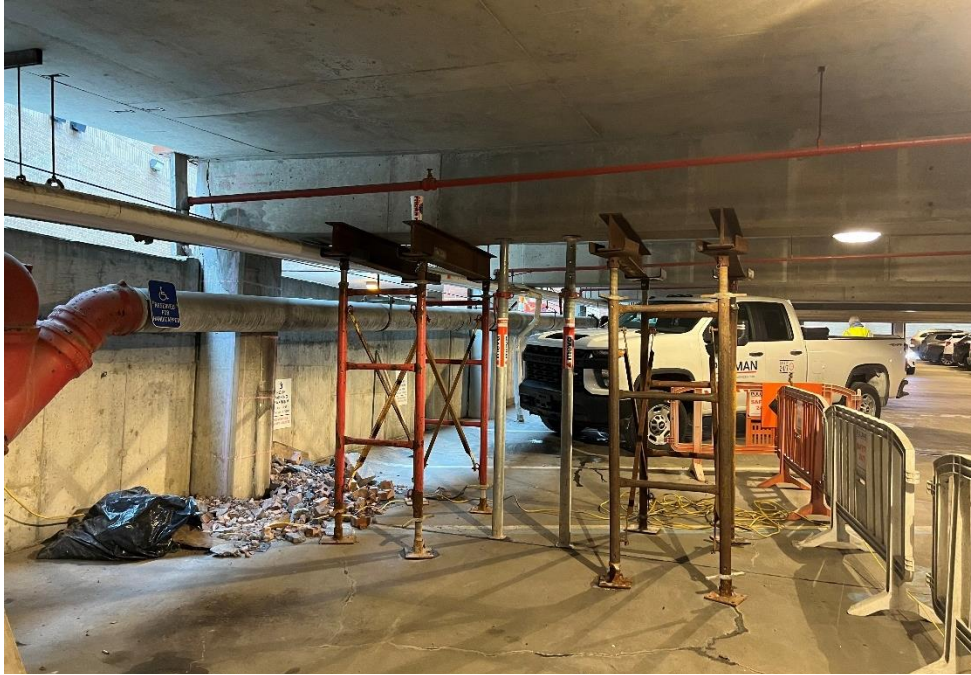
Figure 1. Shoring installed at the west end of the Level 1 beam supported by Column 11A.
