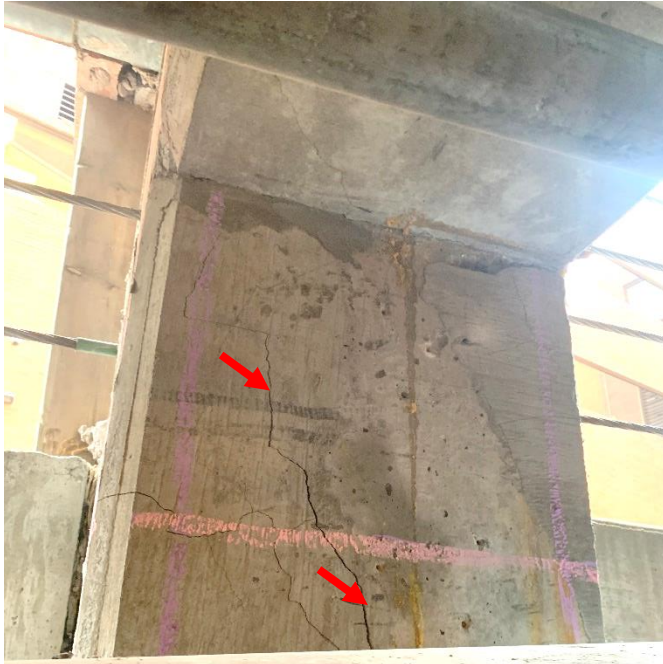
Figure 13. Cracks throughout original concrete at Column 11A.
